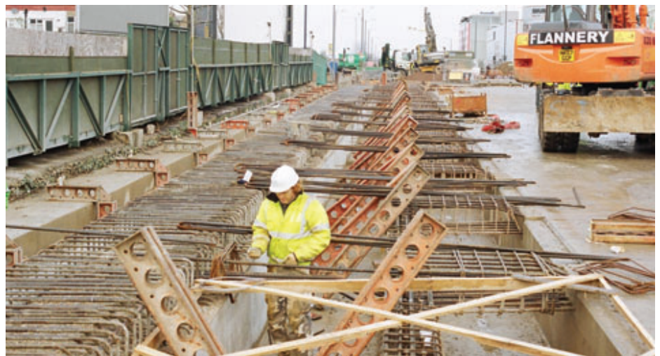
Construction of a services trough for utility diversions at Wales Farm Road Bridge
